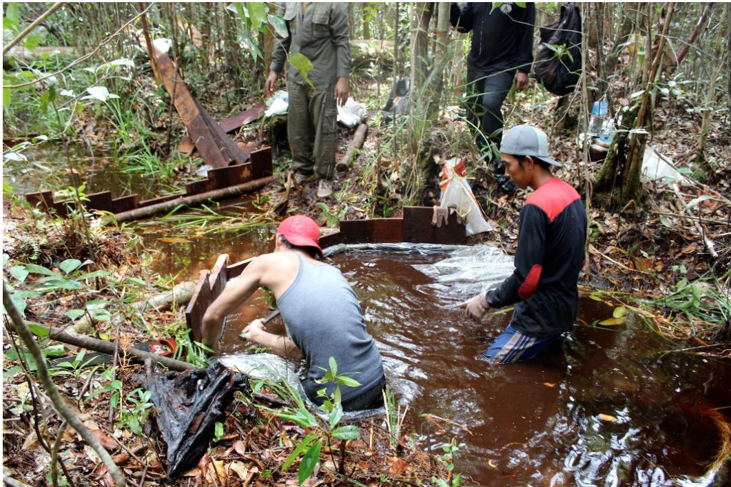
Figure 32: Building a dam in a drainage canal in Sabangau peat-swamp forest in Indonesia. Photo by BNF.
